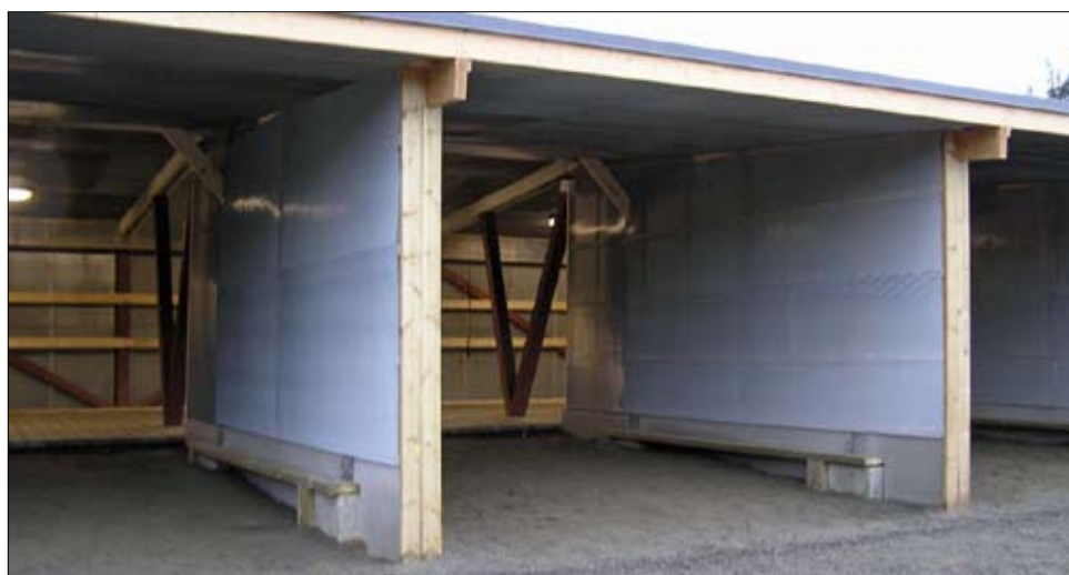
Figure 4. The Parolannummi "noise control" shed. The interior surfaces of the shed and the partition walls were lined with sound absorbing mineral wool covered with protective steel mesh
